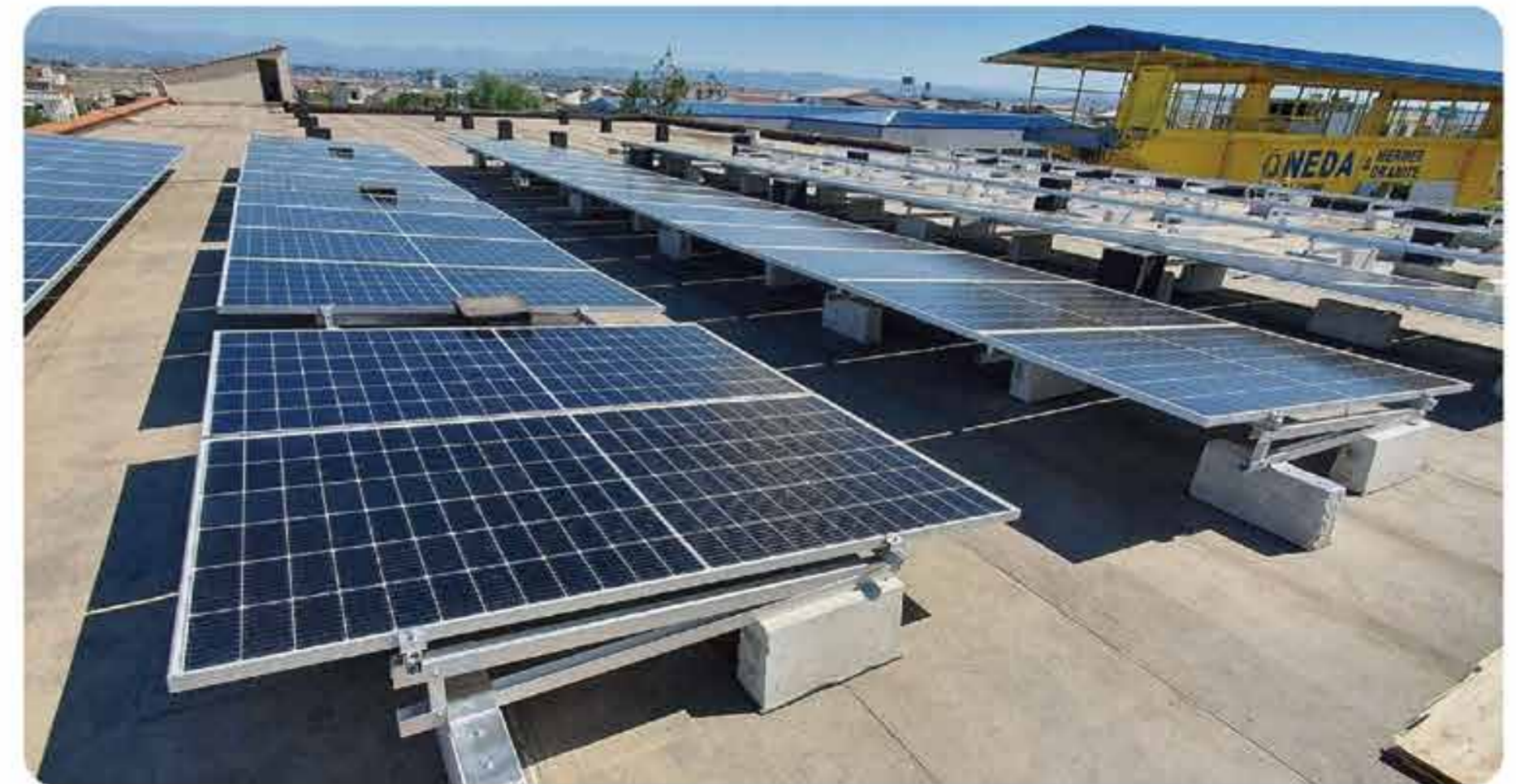
100KW On-grid Solar System in Hungary
