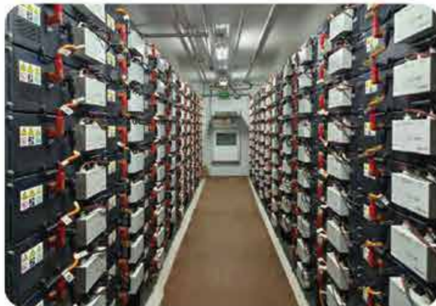
Base station UPS power projects
