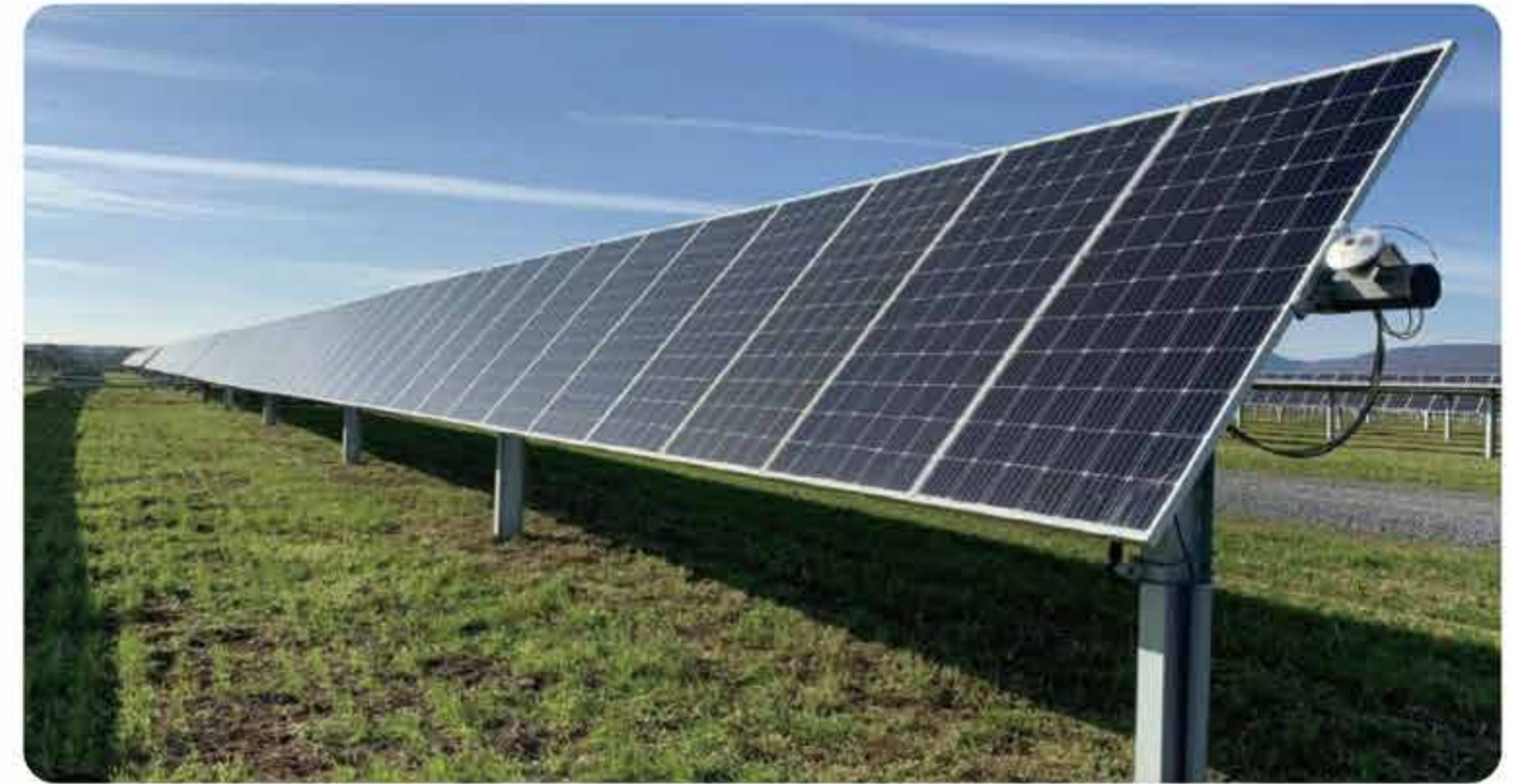
14MW Hy-Grid Solar System
