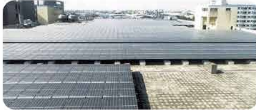
120KW Hy-Grid Solar System In Thailand
