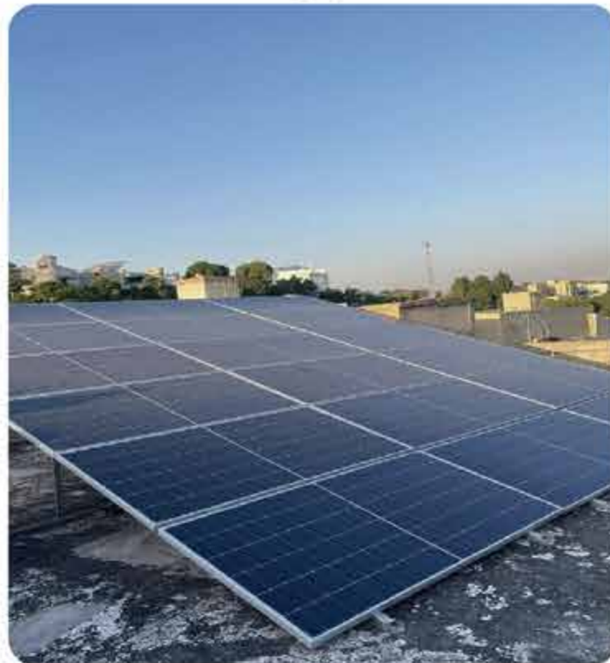
20KW Residential Use in USA
